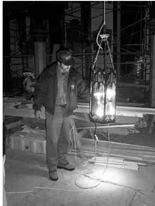
Parishioner, Darrell Knickle conducts light test of restored fixtures.
